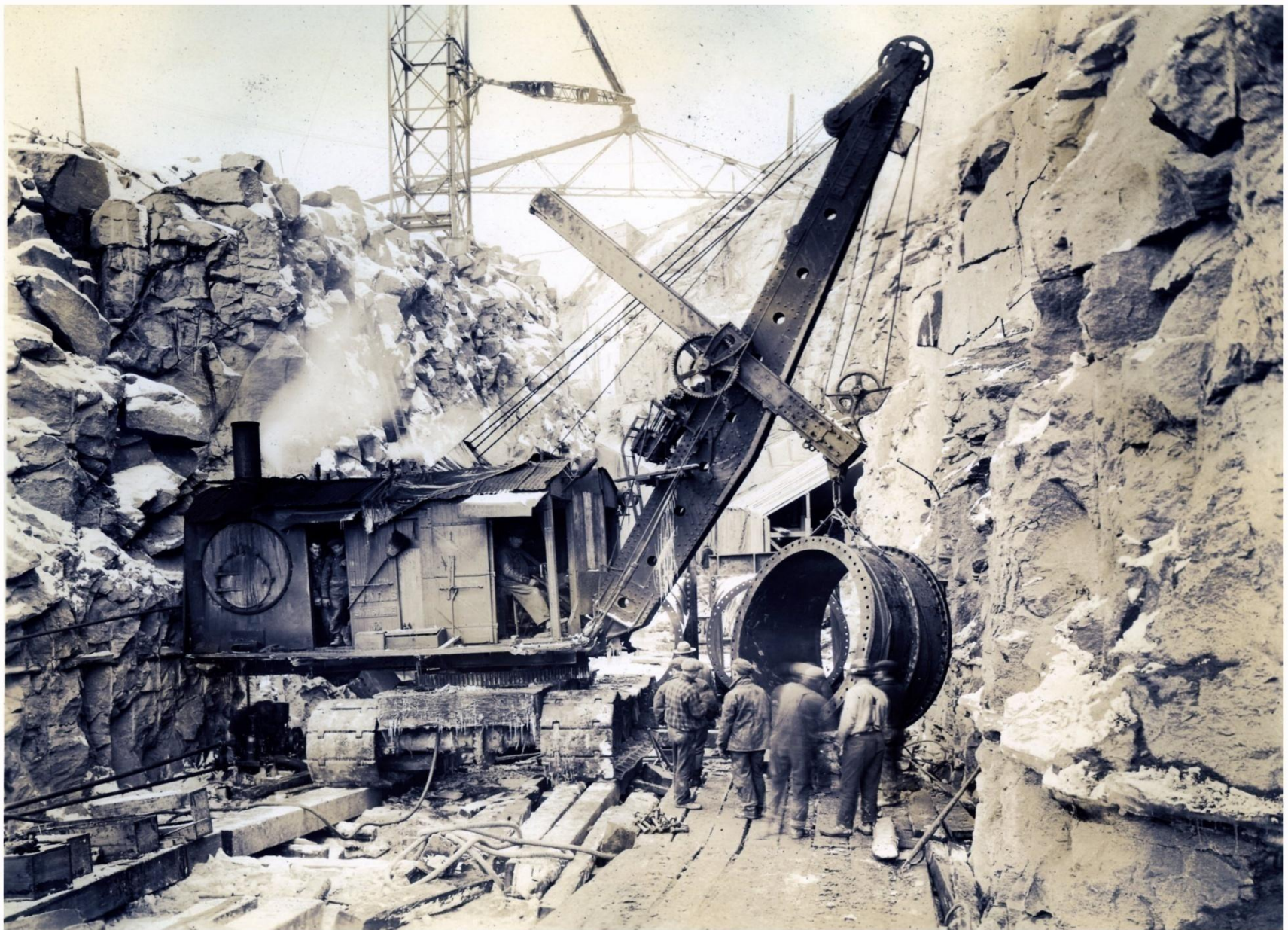
Steam shovel lifting upstream valve extension to swing into final position in outlet channel.
