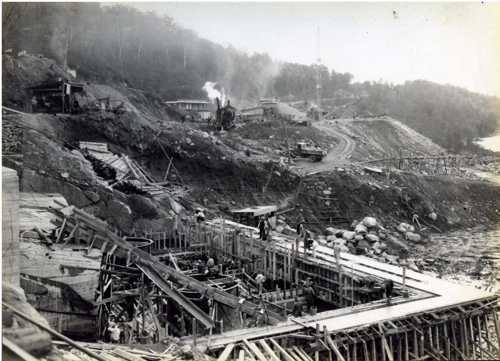
Power House. Looking Southeast across generator section from West side of plant.
