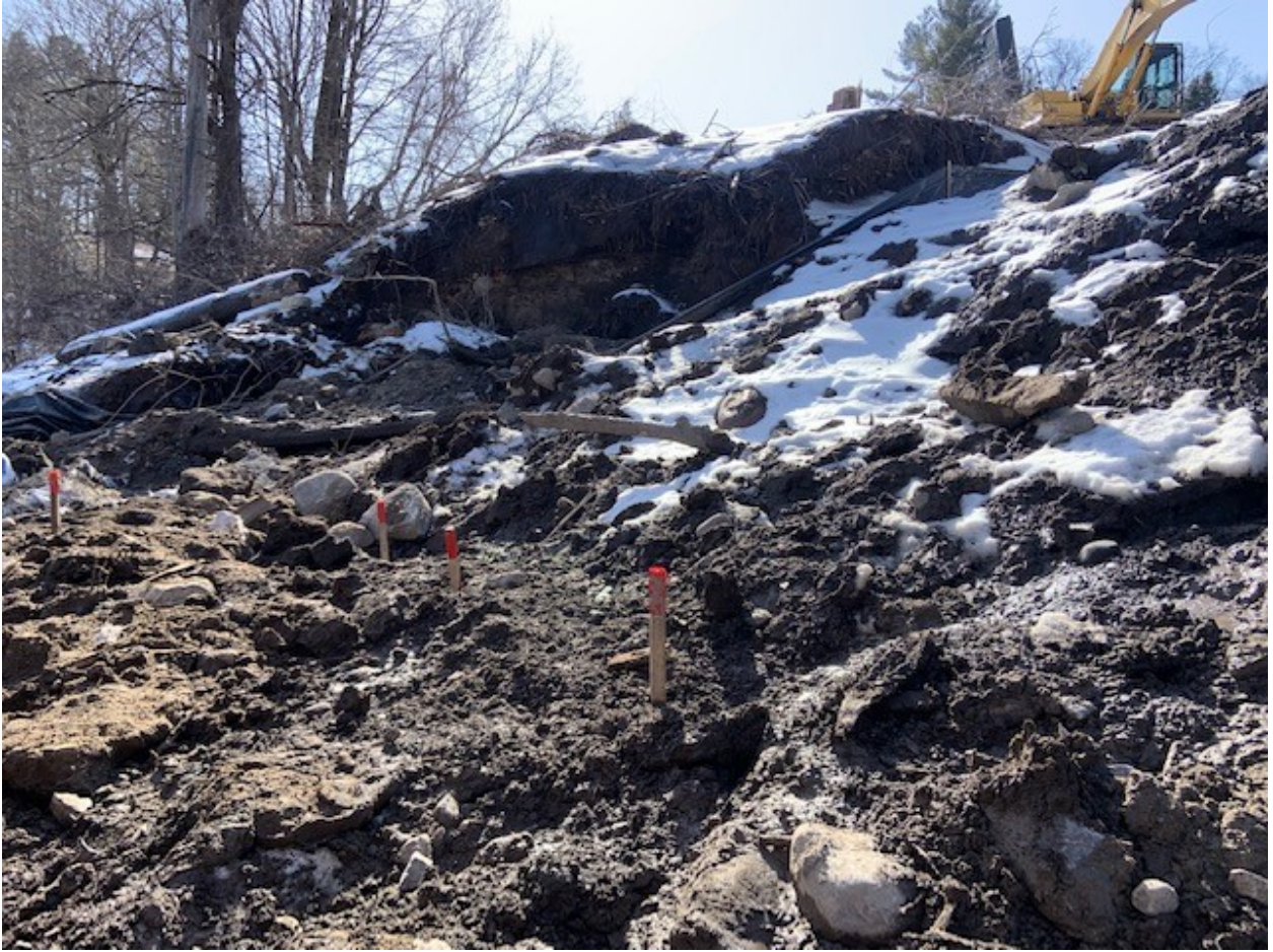
West bank loose soils
