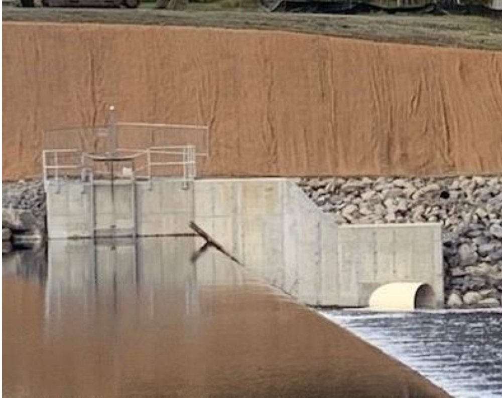
Headwall, Outlet Gate, and Discharge Pipe
